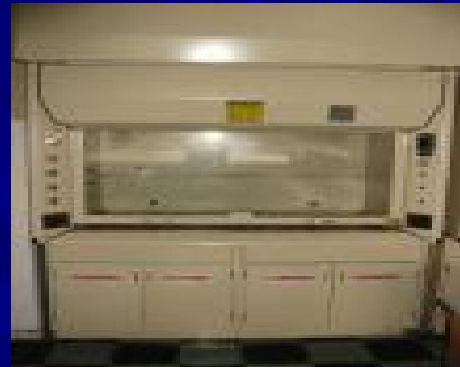
Chemical Fume Hood
