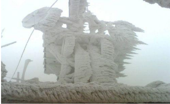
Figure 2 Base station's malfunction in storms, Guangxi, China 2008-02-02 16:26:29
