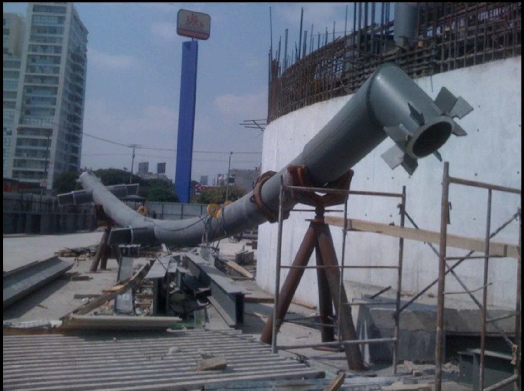
Base Pipe Column
